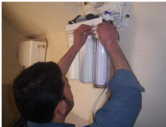
This small water purification system installed by technician Ameer of Yanabi'a Al-Khair Supply Shop (Spring Water Goodness) in Najaf, Iraq, can provide up to 189 liters a day of clean, safe drinking water.
